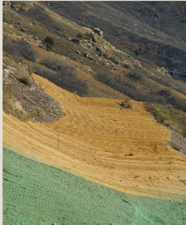
Pipeline reclamation along a steep hillside using both erosion control blankets and a hydraulically applied Bonded Fiber Matrix (BFM). ©Ryan Timoney/Granite Seed Company
