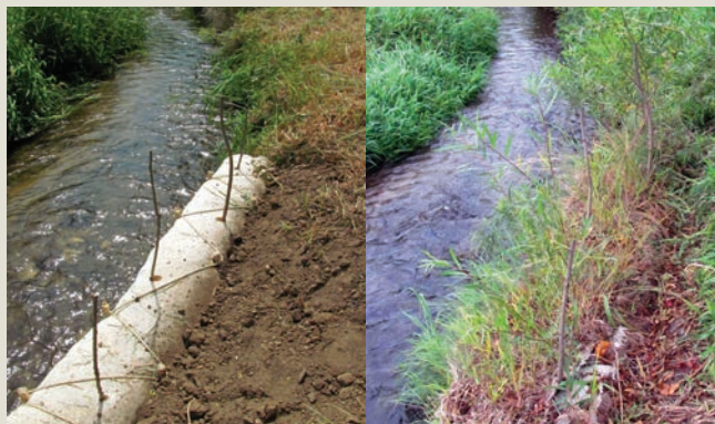
Excelsior fiber erosion control blocks used in a shoreline application with live willow stakes, pictured on the day of installation and three months later. Exterior casing is light in color compared to darker coir logs that can warm water temperatures, which can be detrimental to fish and other aquatic organisms. Functional for 3+ years, but designed to begin biodegrading during the first year as sediment and seed settle into the interior matrix. Also use in other applications such as a replacement for silt fence or for channel filter stations. ©American Excelsior Company
